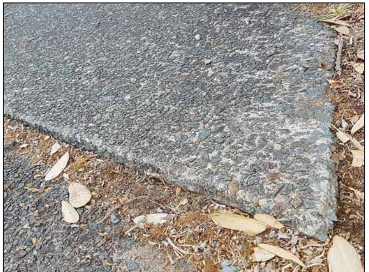
Just one example of the uneven footpaths, which are tripping people up around One Tree Point.
