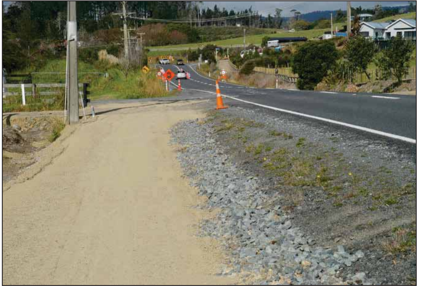
The new section of the Waipu to Waipu Cove cycle and walkway. More funds are needed to take the trail all the way to the Waipu Cemetery
