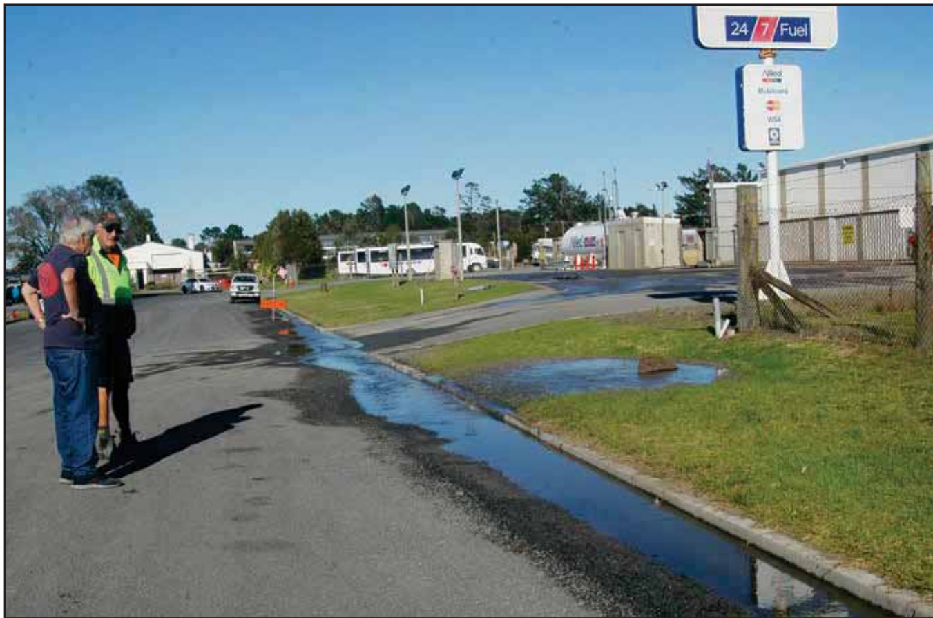
Keith Newey Showing Jules Flight Chairman of the Ruakaka Residents and Ratepayers Association how sewage is spilling out of two manholes in Kepa Rd.
