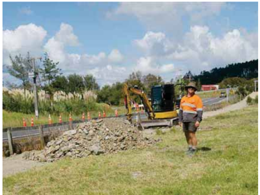
Paul Cowpland at work on the new section of the Waipu to Waipu Cove Cycle and Walkway. The section takes the trail crossing away from the McLean Rd. corner
